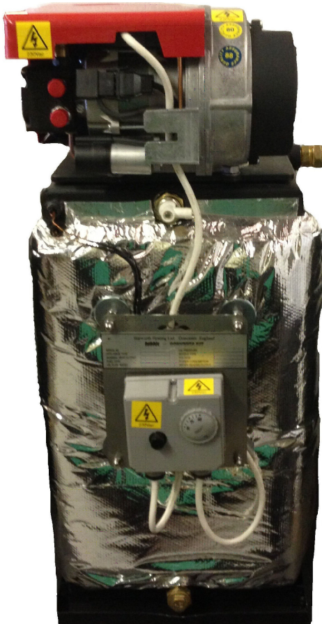
Front View Vertical Boiler
