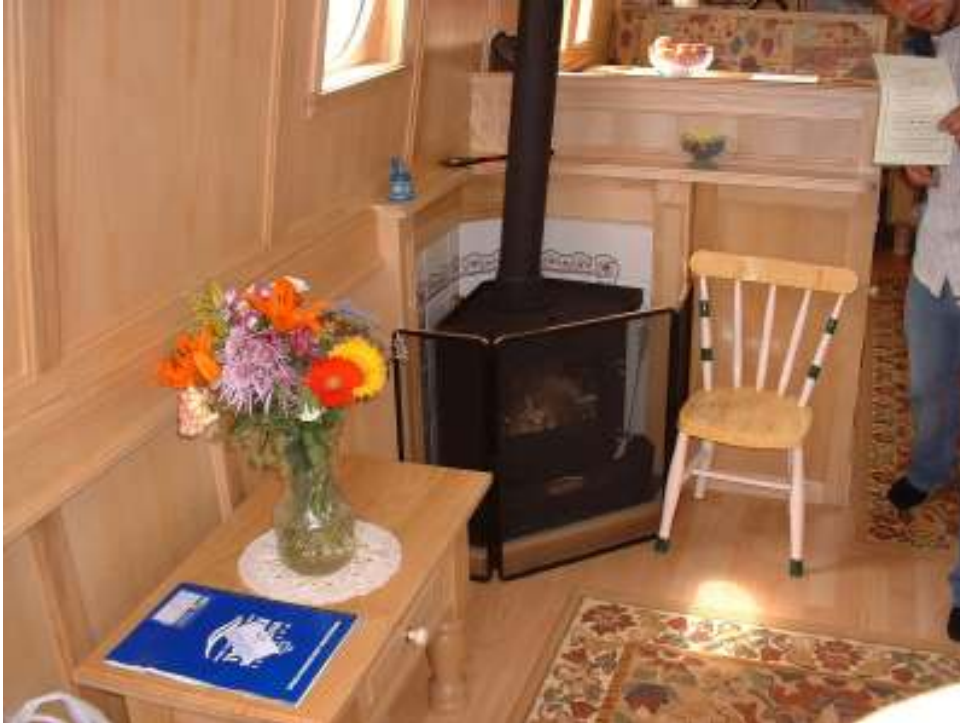
CORNER STOVE IN BOAT (INCORRECT FITTING)
