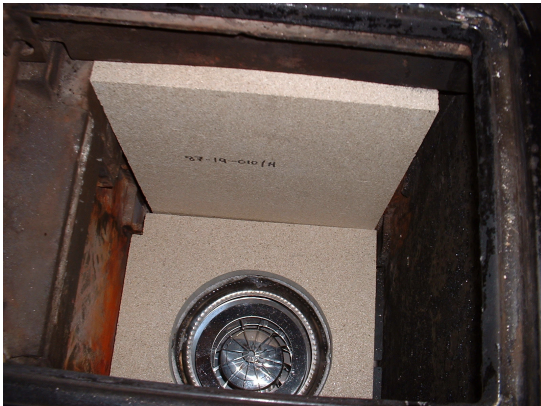
Fit the fuel-loading door masking plate and using it as a template mark out and cut a circle through both boards to accommodate the barometric damper.
