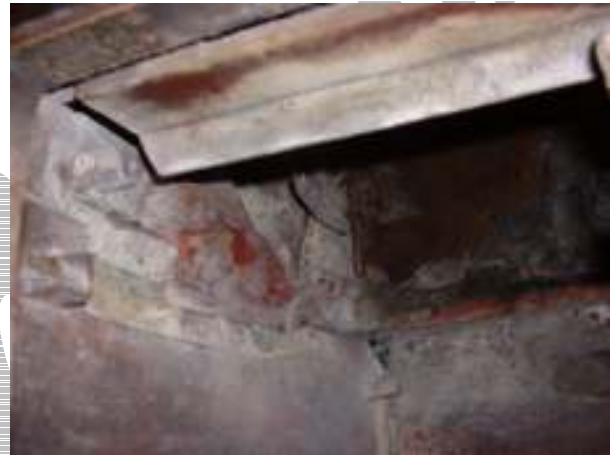
View thro ash pit door showing secondary air casting attached to front plate.
